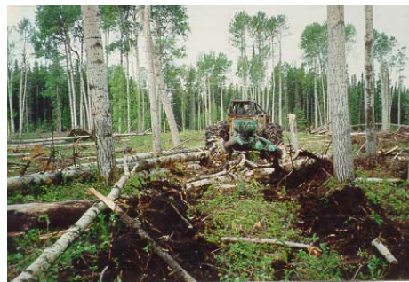
Figure 85. Disc Trencher Each pass of the disc trencher provides 2 rows of planting sites where the organic matter and mineral soil are mixed, creating an excellent site for seedling establishment and growth.
