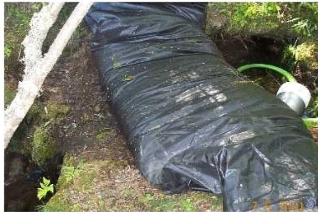
Channel is Totally Sealed Off
