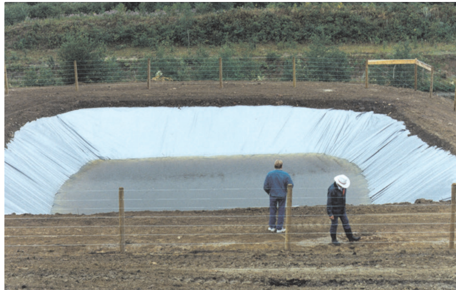
Figure 5-12 Elevated Earthen Reservoir with Woven Polyethylene Liner
