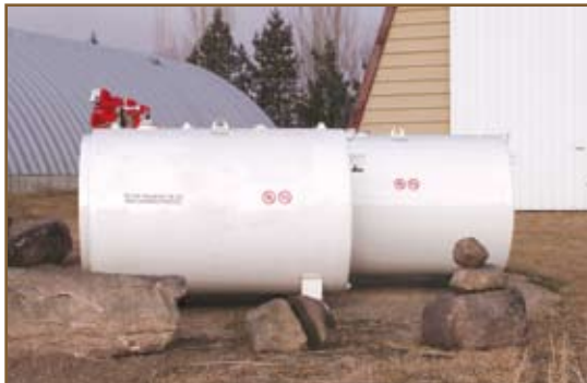
Figure 18: Collision protection using large boulders Photo courtesy of MFP Mohawk Fuel Products Inc. and Scott Stack, 2006
