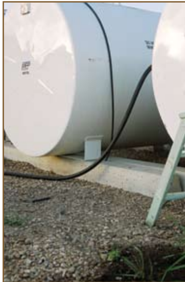
Figure 17: Double walled tanks using concrete supports on firm, compacted gravel Photo courtesy of the Alberta Environmental Farm Plan Company, 2006
