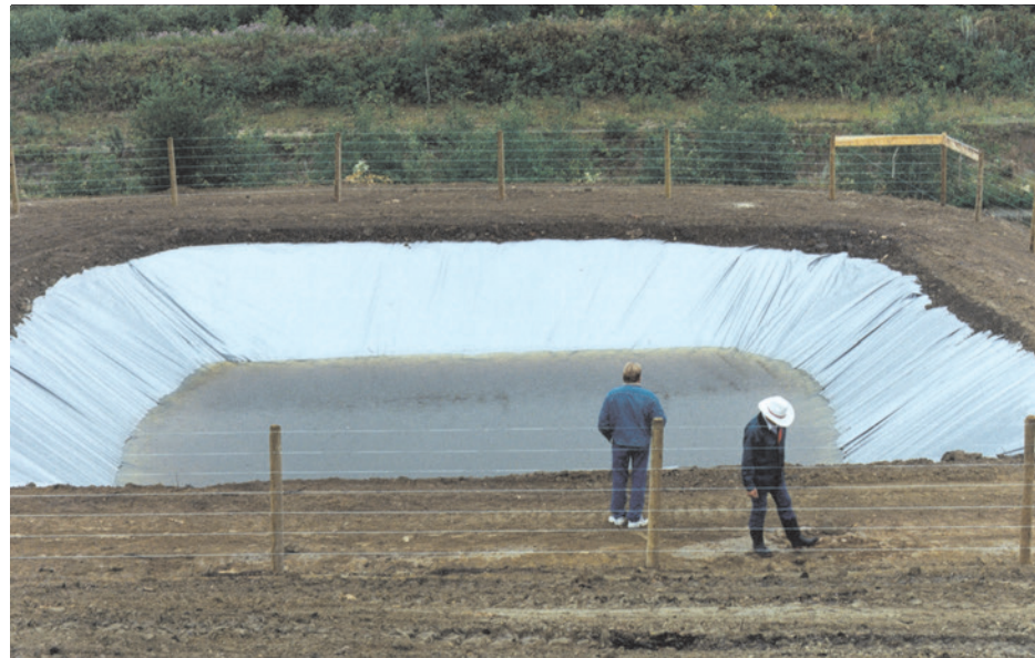
Figure 5-12 Elevated Earthen Reservoir with Woven Polyethylene Liner
