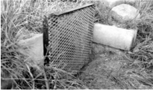
Figure 2. Farm ditch screen bolted to concrete structure
