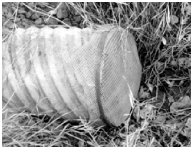
Figure 1. Culvert type screen installed on upstream end of culvert
