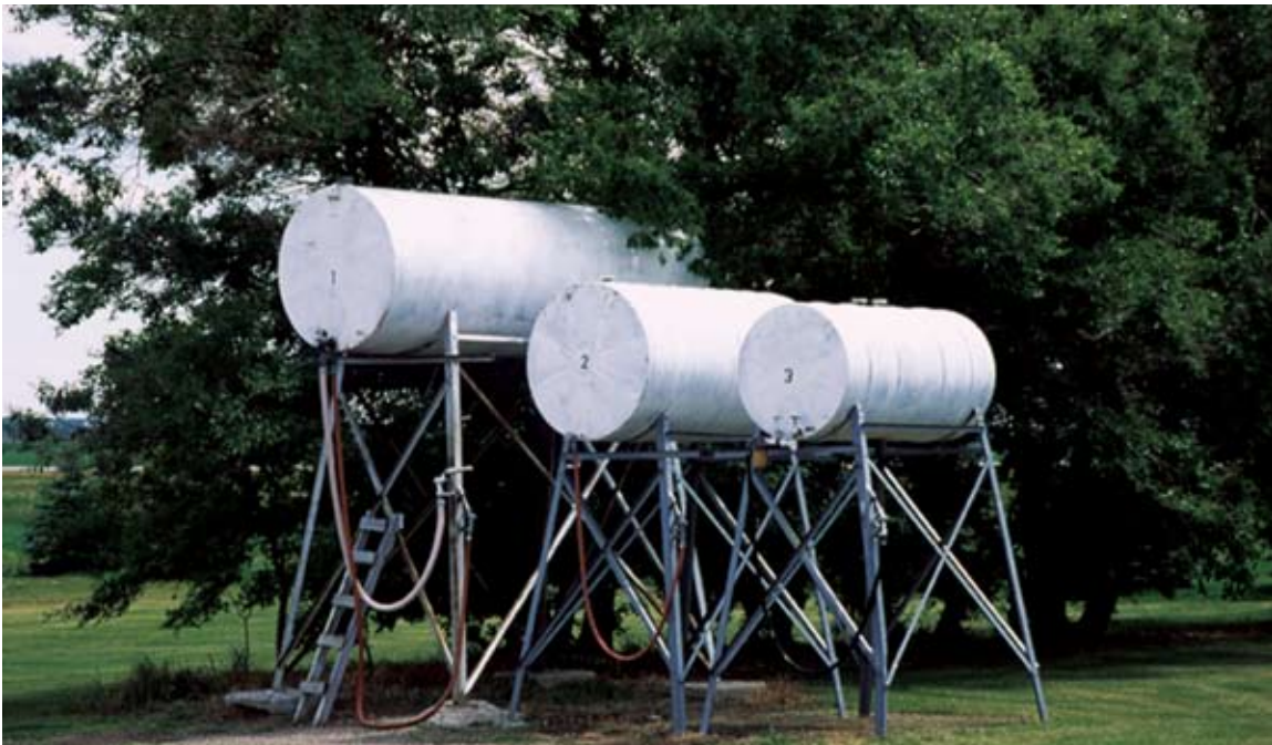
Aboveground or gravity-fed tanks located too close to trees increase fire hazards and damage from fallen trees — Courtesy of AAFRD
